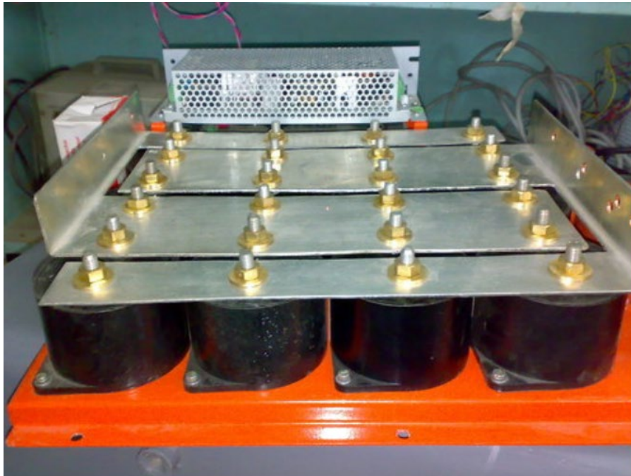
DC-link capacitor bank (in inverter (INV))
